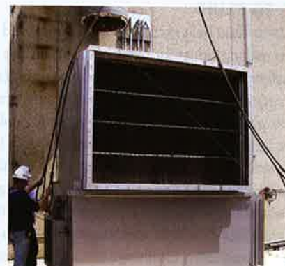
Secondary heat recovery installation.
